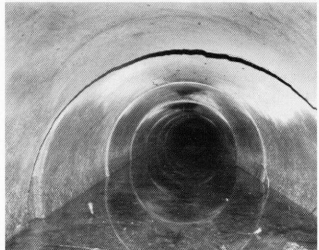
Looking along the flooded emergency exit tunnel at Ardingly Zero Station.
